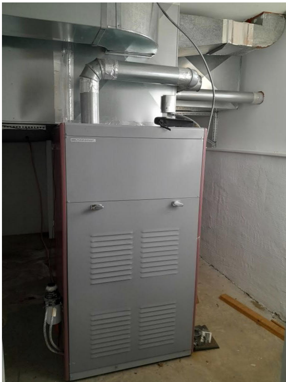
Figure 14 – Existing Oil-Fired Furnace
