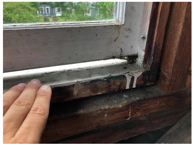
Figure 12 – Large gap between sash and sill.
