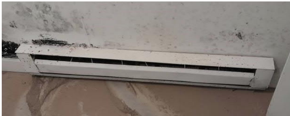
Figure 15 – Existing Electric Baseboard Radiator
