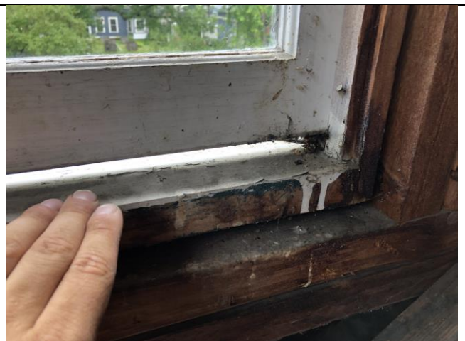
Large gap between sash and sill.
