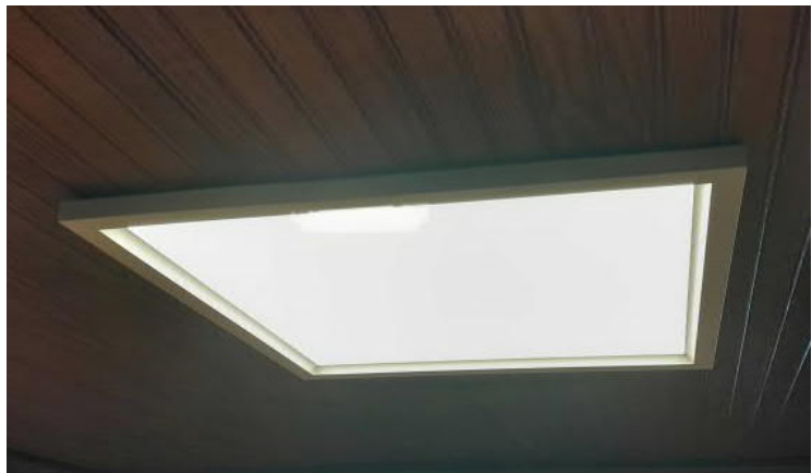
Figure 20 – Existing LED Panel Fixture
