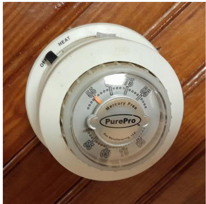
Figure 13 – Existing Non-Programmable Thermostat
